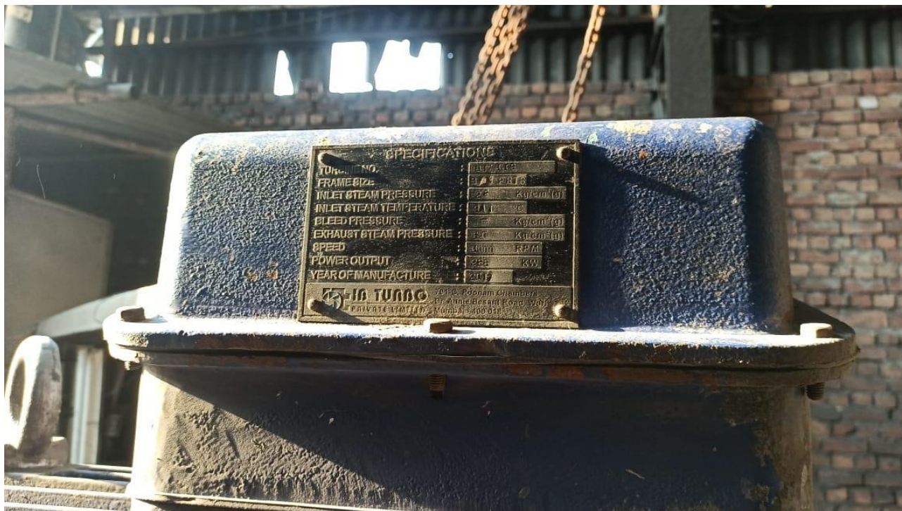
Figure 2: Image of the turbine name-plate details at T. C. Terrytex Limited's Sarsini Plant
